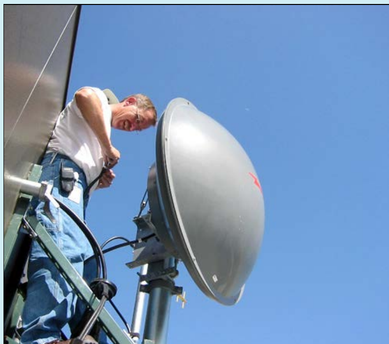
Del Harris, a Network Engineer with NETS, works on a wireless networking antenna linking NCAR/UCAR campuses. NETS is constantly tracking, testing, and deploying new technology as appropriate to provide UCAR users with state-of-the-art networking service. As business continuity has become a higher priority for the organization, NETS has broadened their deployment of MAN wireless technology to provide backup services between all campuses as a disaster recovery measure.
